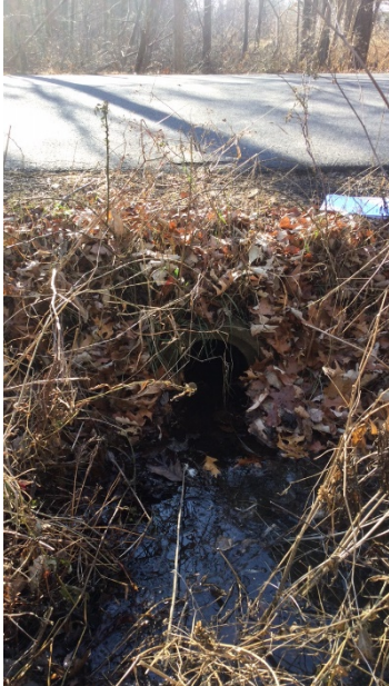
This shows an image of a small 12" diameter culvert passing under a paved road.
